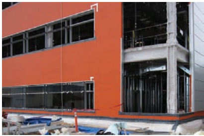
Figure 3. Installation of fully adhered air-barrier (orange membrane) including self-adhering flashing in progress in Central Washington.
